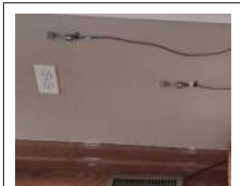
Figure 3. LVDT micro metre displacement gauges placed over an existing vertical drywall crack (above outlet) and null gauge on uncracked drywall (lower right) both below the living room window (molding shown above).
