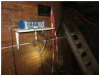
Figure 4. Measuring equipment mounted near the vent, shown is a Tranet Oscilloscope with 8 channels.
